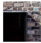
SW Steel framed window Clear glass Location: Windows to fire stair (sprinklered)
